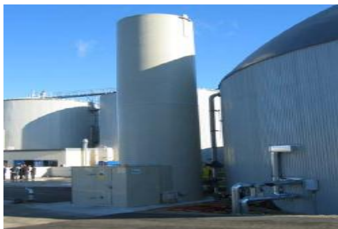
Digester, désulfuration, post-digester
