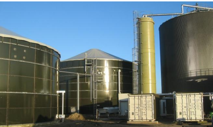
Hydrolyse, post-digester, désulfuration, digester
